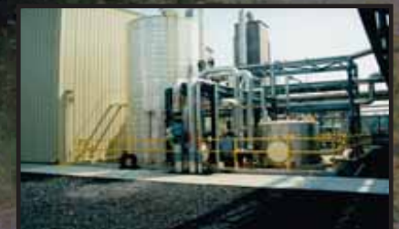
STORAGE TANK OUTSIDE OF WATER TREATMENT FACILITY
