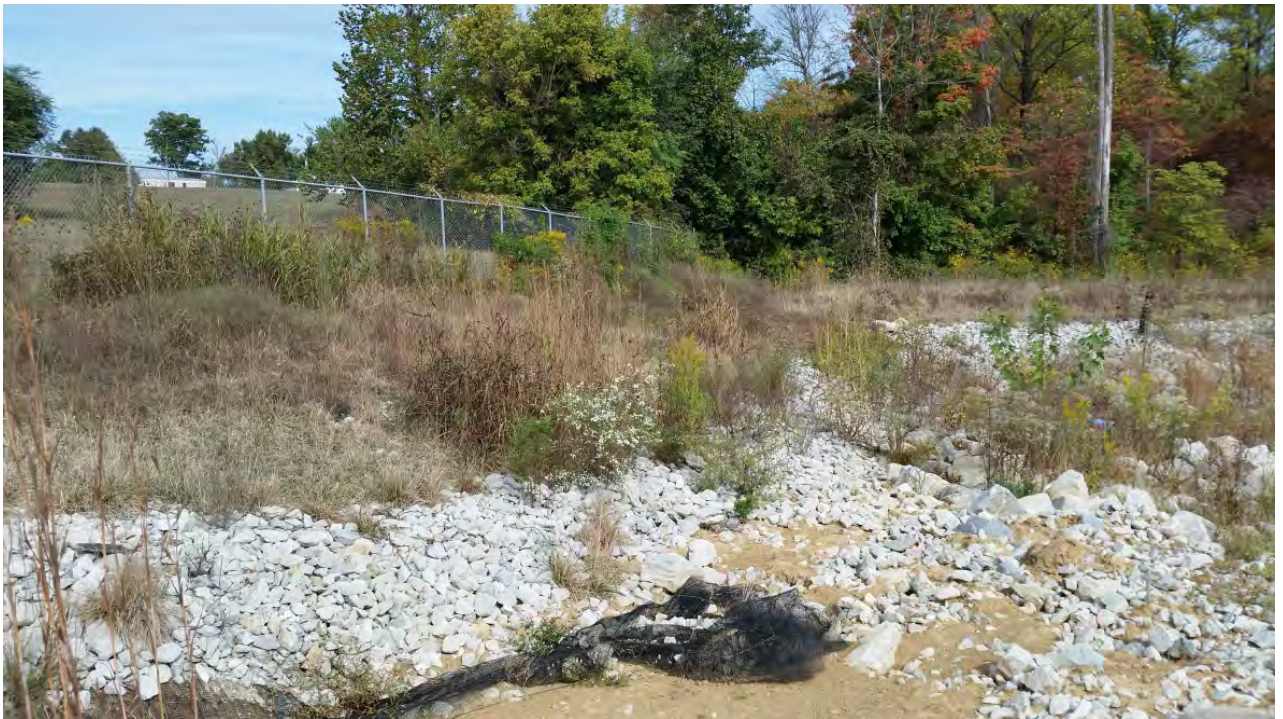
Photo 24: ES6 drainage swale facing west, channel erosion.
