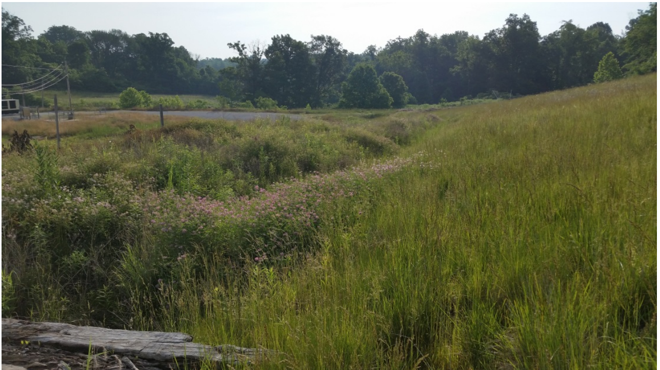
Photo 14: ES14 East Plant Area cover facing northwest
