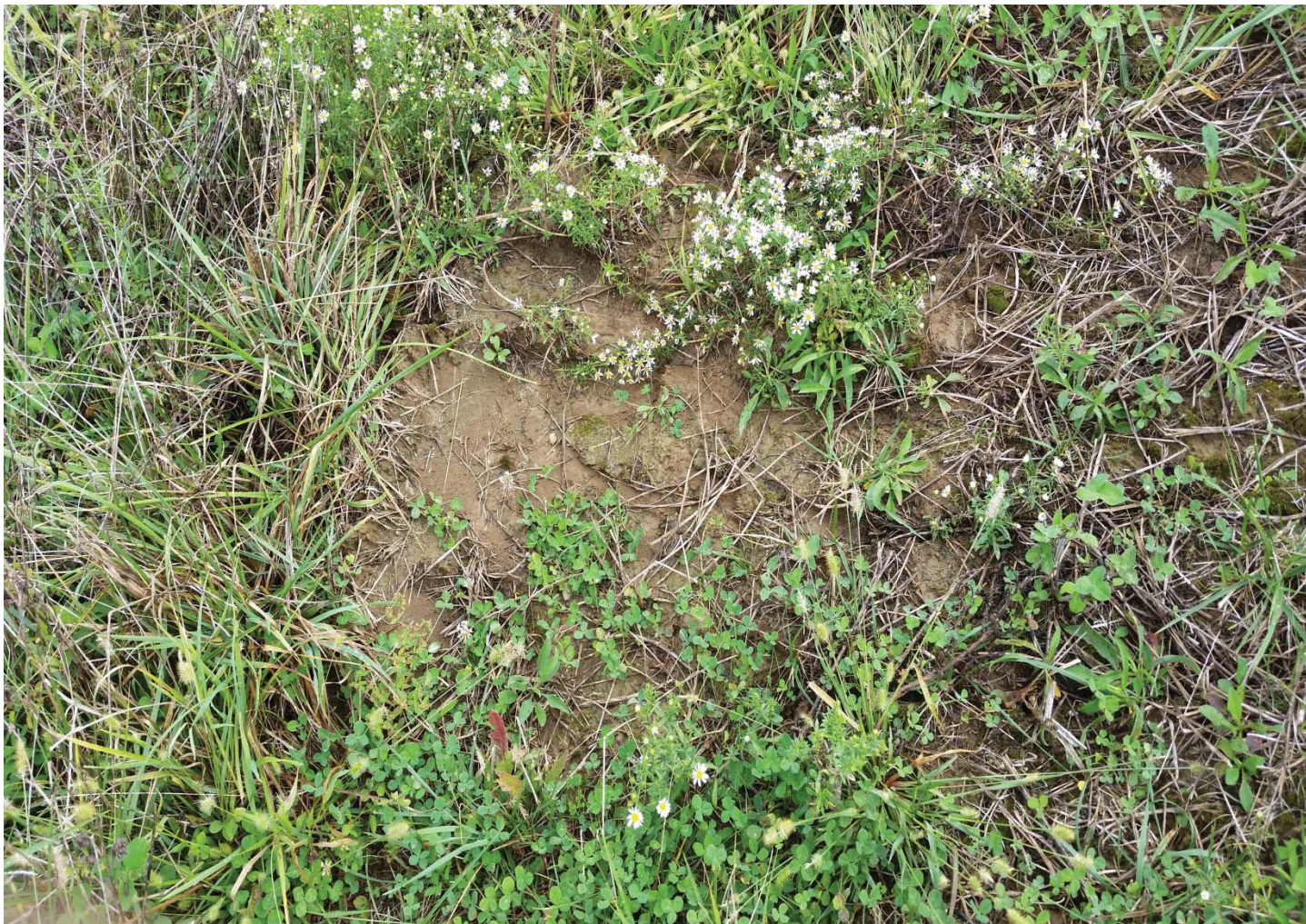
Photo 2: Patchy vegetative growth at EV2 East Plant Area Cover, southwest of ES4
