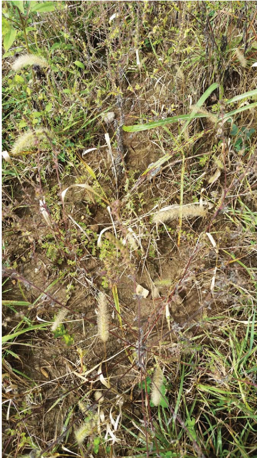
Photo 16: Slight topsoil erosion at EV6 East Plant Area Cover.
